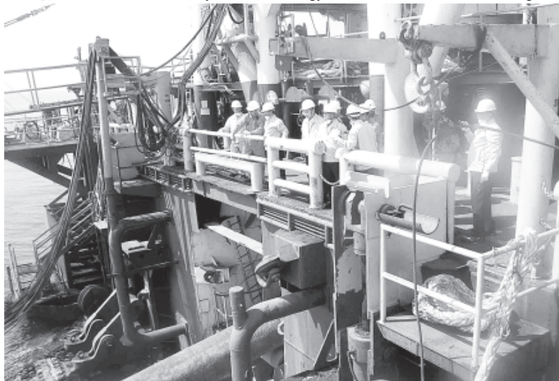
Vice-President Thiha Thura U Tin Aung Myint Oo inspects laying of pipeline from Hyundai HD (60) vessel, part of Shwe natural gas pipeline project.—MNA
