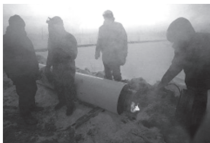
Men work on a pipeline in minus 40 degree celsius temperatures in Novy Urengoi, northern Russia.—INTERNET
