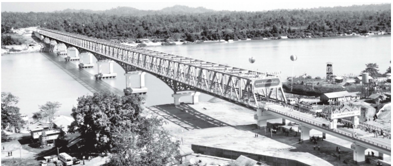
Ayeyawady Bridge (Sinkham) opened as the 11 th of its kind of over 180 feet in the time of the government of the Republic of the Union of Myanmar to hail the 65 th Anniversary Union Day for 2012.—MNA
