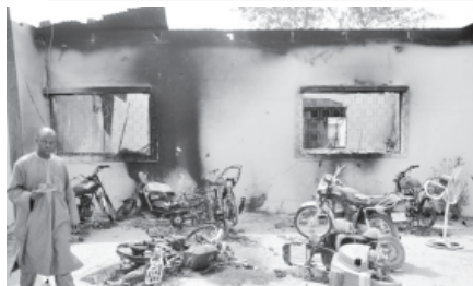
The destroyed police headquarters in Kano, on 21 Jan, 2012.—INTERNET
