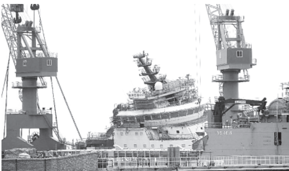
Photo taken on 18 Jan, 2012 shows staff members using cranes to repair the big oilfield workshop at a dock in Nantong City, east China's Jiangsu Province. A workshop worth an investment of 740 million yuan (117 million US dollars) by the China Oilfield Services Ltd (COSL), a leading Chinese oil field service provider, has sunk at a dock during construction on Wednesday. The cause of the accident was under investigation and no environmental pollution was incurred, COSL said.
