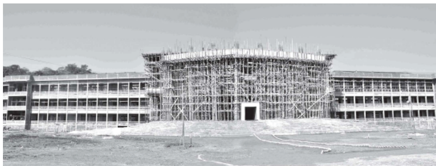
Photo shows progress in construction of three-storey main building at University of Computer Studies (Kalay).—MNA
