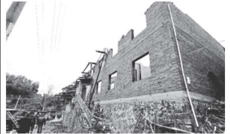
Photo taken on 16 Jan, 2012 shows the damaged building in Shangdian Village of Jian'ou City, southeast China's Fujian Province, on 16 Jan, 2012. The fire broke out on about 4 am on Monday here, destroying two buildings and leaving nine people dead, one injured and one still missing. The cause of the fire is still under investigation.—XINHUA
