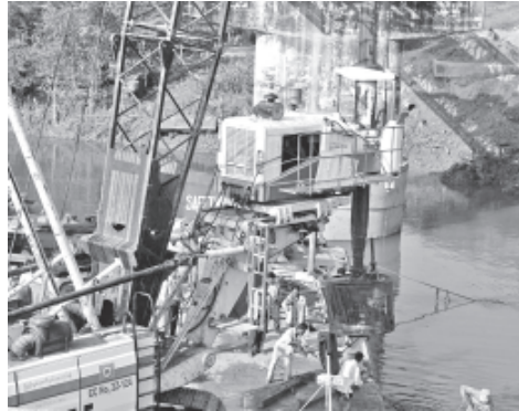
NAY PYI TAW, 14 Jan—Union Minister for Construction U Khin Maung Myint inspected repair work on Nay Pyi Taw-Taungnyo-Myothit-Kanpya (Magway) road and measures for prevention of Sun Creek Bridge against erosion on 12 January. Next, he inspected Minbu-Padan-A road expansion and paving of gravels.
