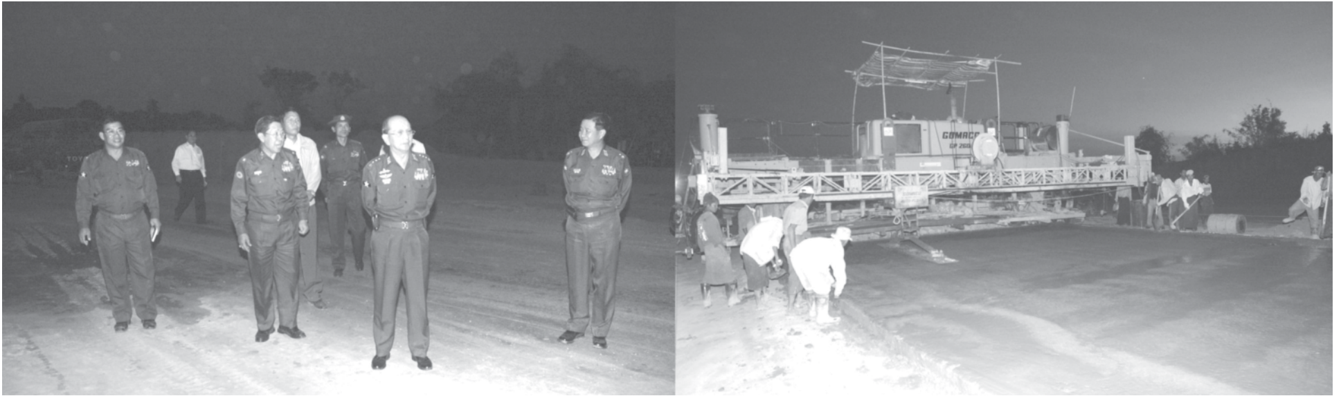
Prime Minister General Thein Sein looks into progress of construction of earth road and paving concrete along Yangon-Mandalay Highway.—MNA
