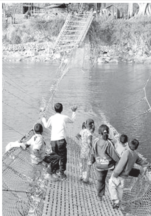
Nepalese children stand on a collapsed bridge over the Bheri River, in the Surkhet district of western Nepal, on 26 Dec, 2007. Sixteen people were killed and 25 still missing from the collapse of a bridge in west Nepal, police said on Thursday, calling it a “miracle” the toll was not higher.—INTERNET
