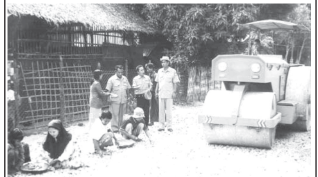
ROAD REPAVED: Twantay Township Development Affairs Committee is repaving Bayintnaung Road spending the cash donated by wellwishers. On 12 December, Director U Khin Maung Cho of Yangon Division Development Affairs Committee and Deputy Superintending Engineer U Zaw Myo Aung inspect tarmacking of the road. — TOWNSHIP DAC
