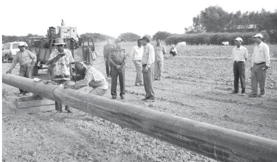
Minister Brig-Gen Lun Thi inspects laying gas pipe line linking Magway, Pyawbwe, Taunggyi and Pinpet. — MNA
