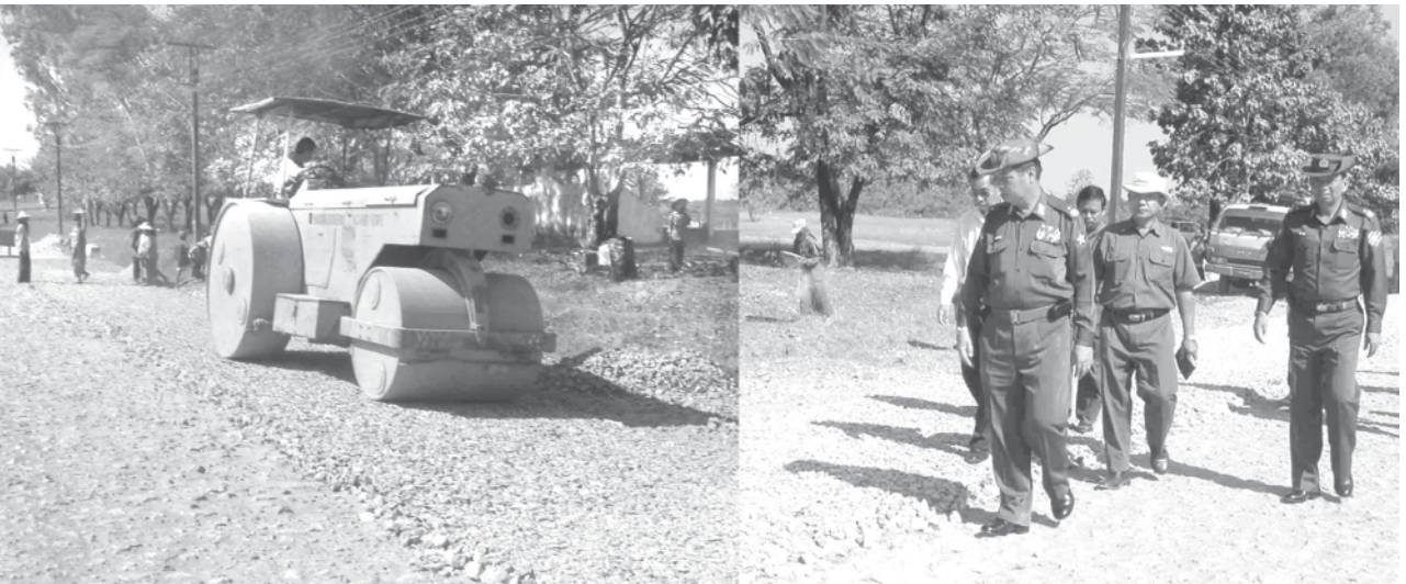
Maj-Gen Tha Aye of Ministry of Defence inspects road works on Mawlamyine-Hpa-an Road. — MNA
