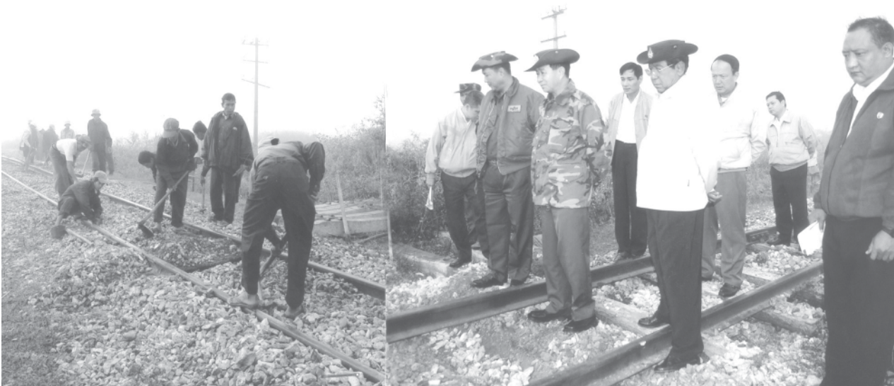
Minister for Rail Transportation Maj-Gen Aung Min inspects upgrading tasks of Yangon-Pyay railroad.— MNA
