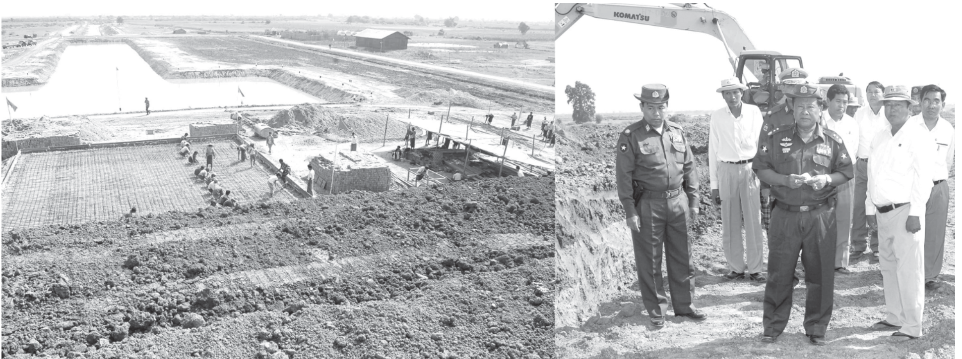
Lt-Gen Ye Myint of Ministry of Defence inspects river water pumping project for supplying water to Meiktila Plain. — MNA
