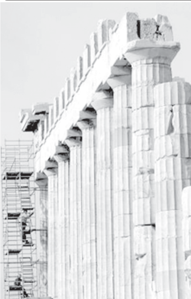
Construction workers are seen atop scaffoldings during restoration work at the ancient temple of Parthenon on the hill of Athens' Acropolis November 27, 2007. — INTERNET
