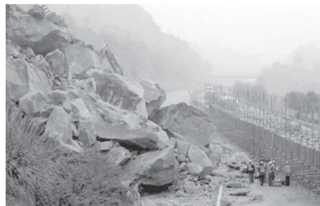
Workers clear debris at a landslide site of Yuyi highway (Chongqing to Yichang city of Hubei Province), in southwest China's Chongqing municipality on 26 Nov, 2007.—INTERNET
