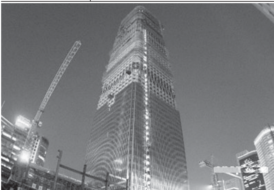
The roof of the main building of the third-phase construction project in Guomao, or China World Trade Center, a major business area in Chaoyang District, Beijing, has been capped on 29 Oct, 2007.—INTERNET
