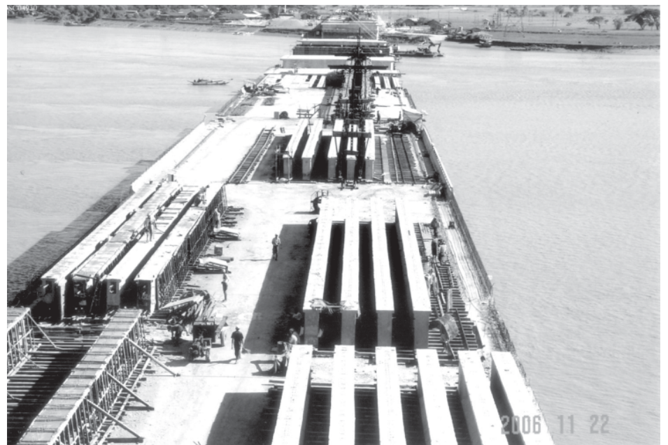
One hundred and ten feet long PC beams (girders) are laid on the main bridge.
