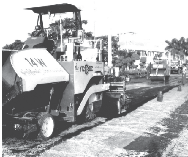
Mayor Brig-Gen Aung Thein Lin inspects roadworks on Ayeyawun Road in Thakayta Township. — MNA
