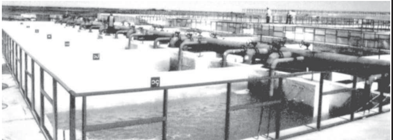
Tanks for urban water supply in Yangon Division.
