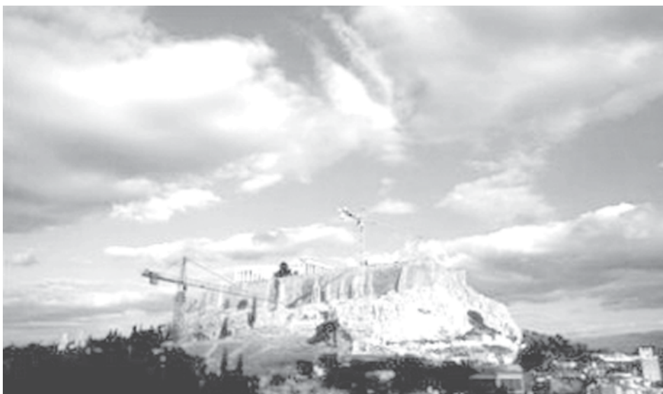
Cranes are seen at the foothills of the Acropolis during a transfer operation of artefacts from the Acropolis to a new location some 400 metres away in Athens on 14 Oct, 2007.
