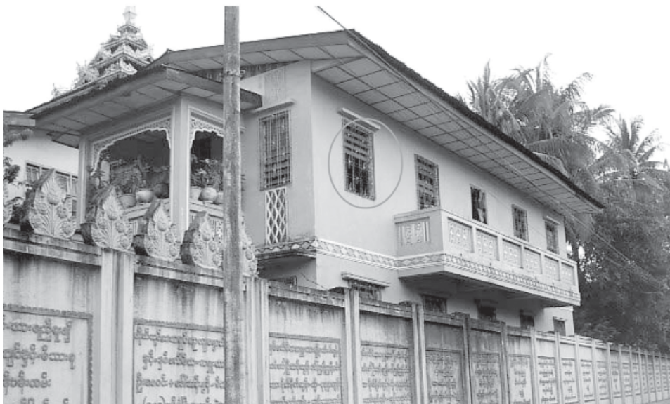
Photo shows a damaged window pane of Khemikayon Hostel in Kyakhatwaing Monastery. — MNA
