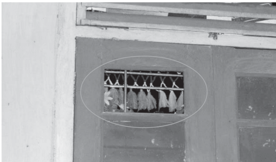
Photo shows a damaged window pane of Ottara Hostel in Kyakhatwaing Monastery. — MNA
