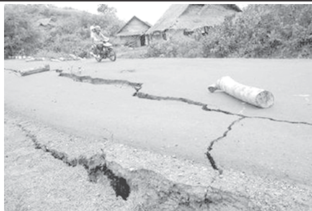
A crack runs down the centre of a street in Lais, after an earthquake rocked Sumatra Province, on 13 Sept, 2007. —INTERNET
