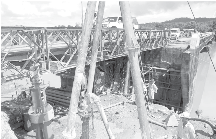
Lt-Gen Khin Maung Than looks into construction of Shwehlay Bridge on Taungup-Thandwe Road. — MNA
