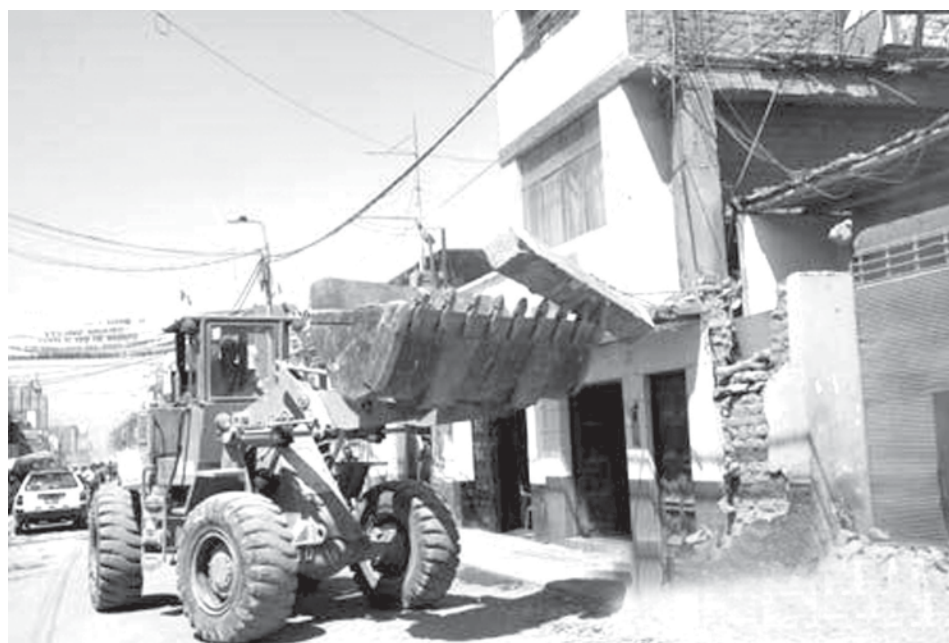
A bulldozer demolishes a house destroyed by quake in Ica, south Peru, on 21 Aug, 2007. A quake measuring 7.5 on the Richter scale hit south Peru on 15 Aug. The Peruvian government has planned to employ some 8,000 people to clear the rubble and reconstruct three of the worst-hit cities, namely Pisco, Ica and Chincha, Peruvian President Alan Garcia has said.—XINHUA
