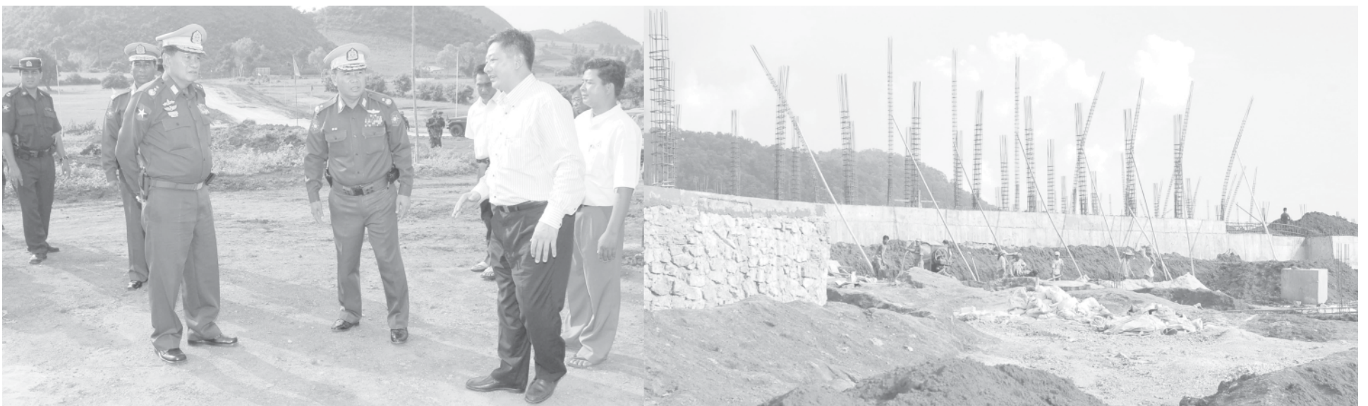
Lt-Gen Kyaw Win of Ministry of Defence inspects construction of three-storey main building for University of Computer Studies in Lashio. — MNA
