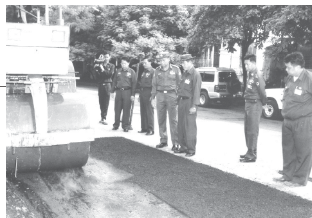
Mayor Brig-Gen Aung Thein Lin inspects repairing of Lower Kyimyindine Road in Ahlon Township on 21 August. — YCDC
