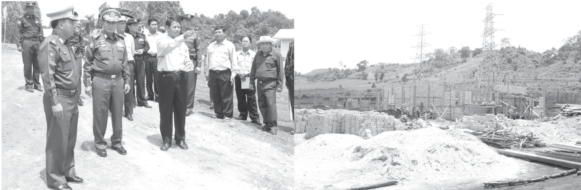
Lt-Gen Kyaw Win inspects installation of 230-KV cables and construction of sub-power stations in Namtu Township. — MNA
