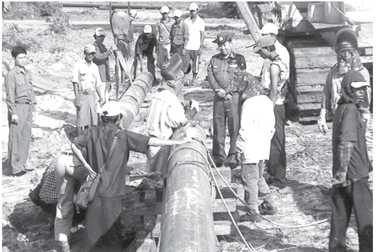
Minister Brig-Gen Lun Thi inspects laying of 14-inch diameter natural gas pipelines from Magway to Pyawbwe. — MNA
