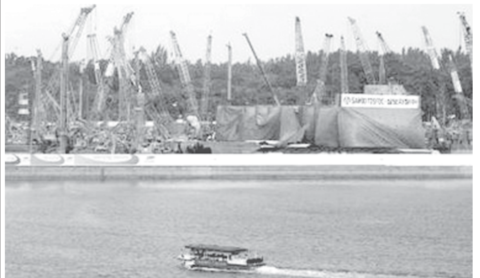
A boat passes the construction site of the Marina Bay Sands casino in Singapore, on 10 Aug, 2007. Singapore's economy expanded at a forecast-beating annualised 14.4 percent in the second quarter, its fastest pace in two years, but the government warned that the turmoil in international credit markets could hurt growth.—INTERNET
