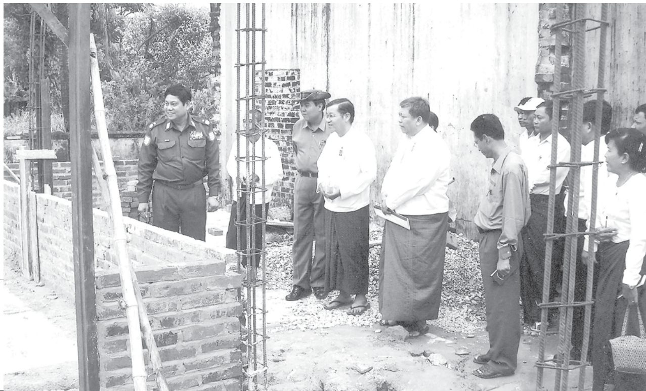
Minister Maj-Gen Htay Oo inspects construction of school building at BEHS in Duya Village in Hinthada Township.
