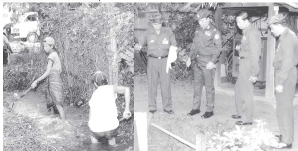
Mayor Brig-Gen Aung Thein Lin oversees unblocking of a drain in Tamway Township. — YCDC
