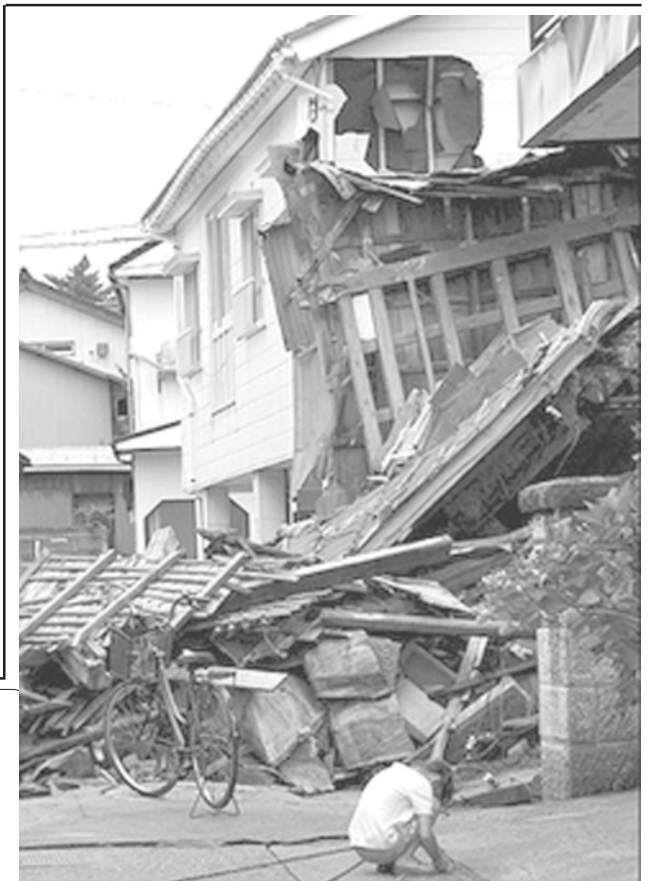
A girl plays in front of damaged houses in Kashiwazaki, on 18 July 2007. Japan on Friday asked businesses to save on energy during peak hours this summer after a powerful earthquake led to the closure of the country’s largest nuclear power plant, officials said. — INTERNET
