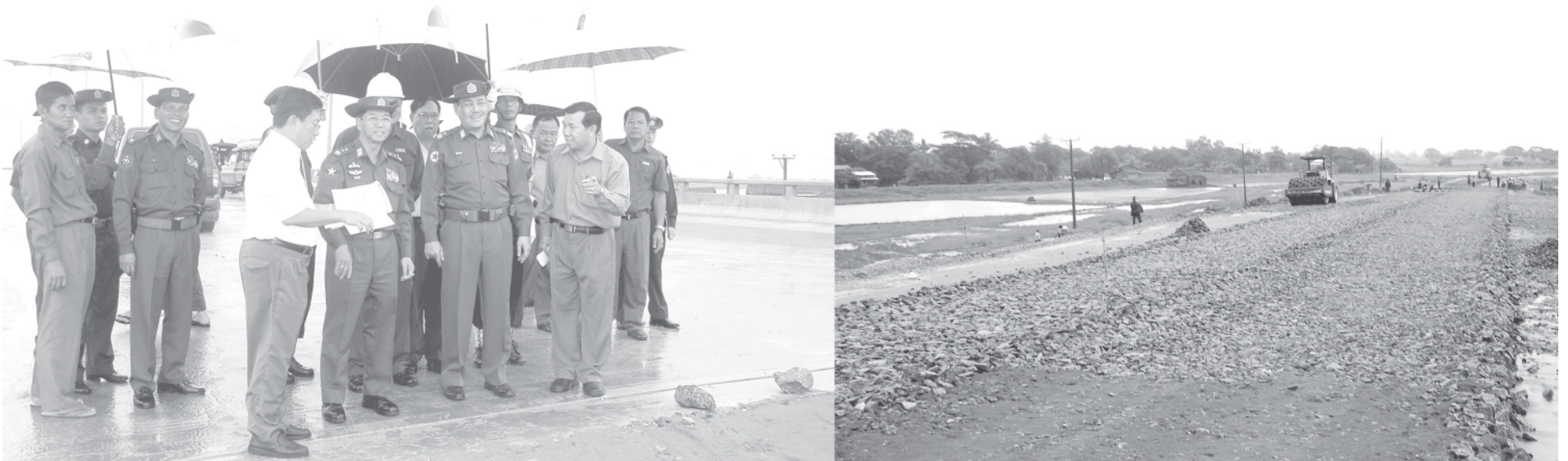
Lt-Gen Myint Swe of Ministry of Defence inspects progress of approach road to Dagon Bridge in Dagon Myothit (Seikkan) Township. — MNA
