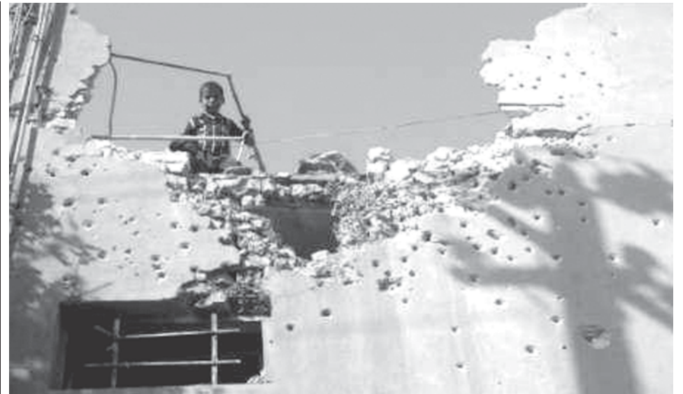
A boy stands on a damaged rooftop after a raid by the US military in Baghdad's Sadr City on 30 June, 2007. The US military said it killed about 26 militants believed to have ties to "Iranian terror networks" in the early hours of Saturday in the Baghdad Shi'ite stronghold of Sadr City. —INTERNET
