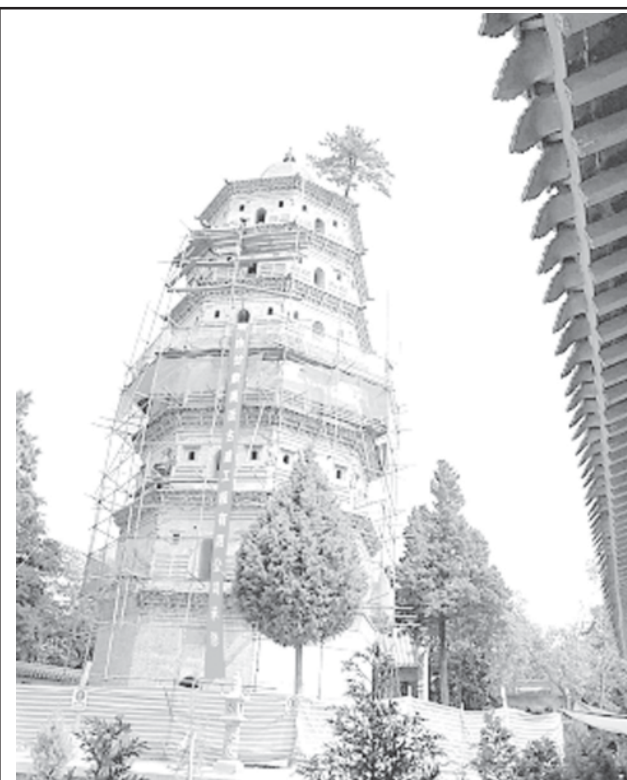
Repairs have begun on the famous Lingkong (high-up) Tower on the Kongtong Mountain in northwest China's Gansu Province, which has long been nicknamed China's "leaning tower in Pisa" as it is famed for being tilted northward. —INTERNET
