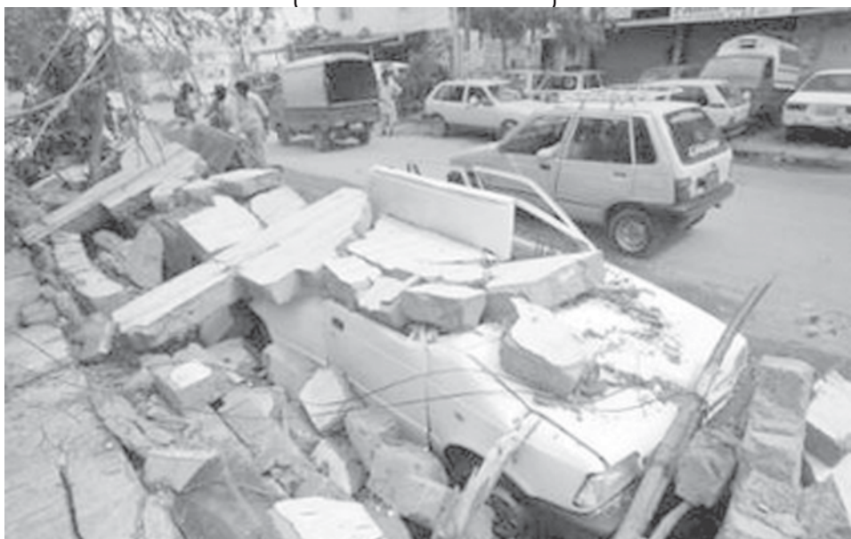
A car is buried under a collapsed wall after thunderstorms and rain in Karachi on 24 June, 2007. INTERNET
