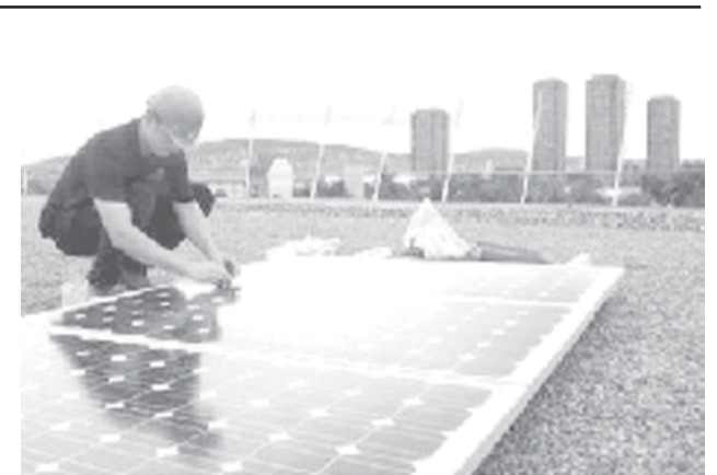
A worker installs solar cells at the new soccer stadium Letzigrund in Zurich, on 21 June, 2007. The building site will be finished in August 2007. — INTERNET
