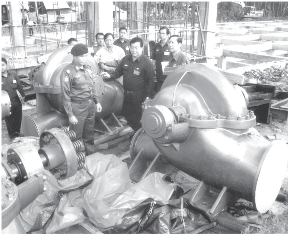
Mayor Brig-Gen Aung Thein Lin inspects pumps in Yeku Water Pumping Station in Mayangon Township.—YCDC
