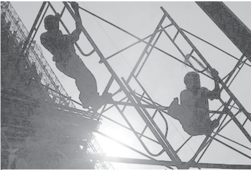
Indonesian construction workers put up scaffolding next to a building site on 15 June, 2007, in Jakarta, Indonesia.—INTERNET
