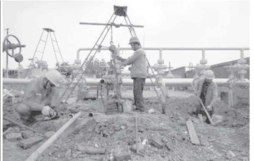
Workers install pipes at a gas exploration site in Guang'an, Sichuan Province, on 13 June, 2007. China's industrial output surged 18.1 percent in May from a year earlier, beating market forecasts and hardening the case for further policy tightening to tamp down the world's fastest-growing major economy.—INTERNET
