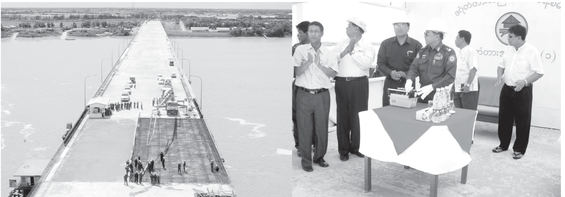
Minister Maj-Gen Saw Tun presses the button key of concrete pump truck to start laying of concrete on the floor of Dagon Bridge in Dagon Myothit (Seikkan) Township.—CONSTRUCTION
