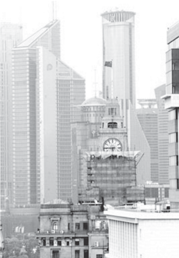
Photo taken on 11 June, 2007 shows the bell tower of the Shanghai Customs in maintenance in the Bund of Shanghai, east China. The bell tower, which was built in 1927 and considered as a landmark in the Bund for 80 years, stopped running on 1 June, for a 4-month maintenance. —XINHUA
