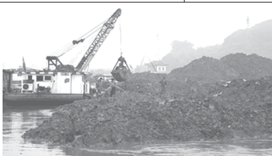
A cofferdam of Dushan flood control works is breached to discharge water of Taihu lake in Wuxi, east China’s Jiangsu Province, on 1 June, 2007. Breaches were made on some cofferdams of China’s third-largest Taihu lake to sluice water polluted by an blue-green algae bloom. Water authorities had also diverted the Yangtze River to dilute the lake water. — XINHUA
