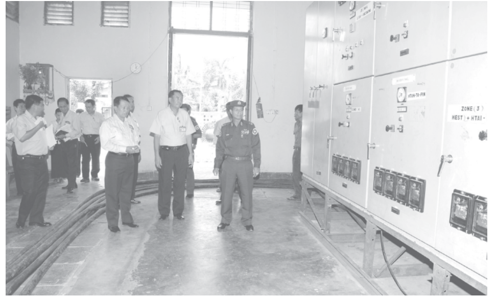
Minister Maj-Gen Khin Maung Myint inspects Hlinethaya sub-power station in Hlinethaya.—MNA
