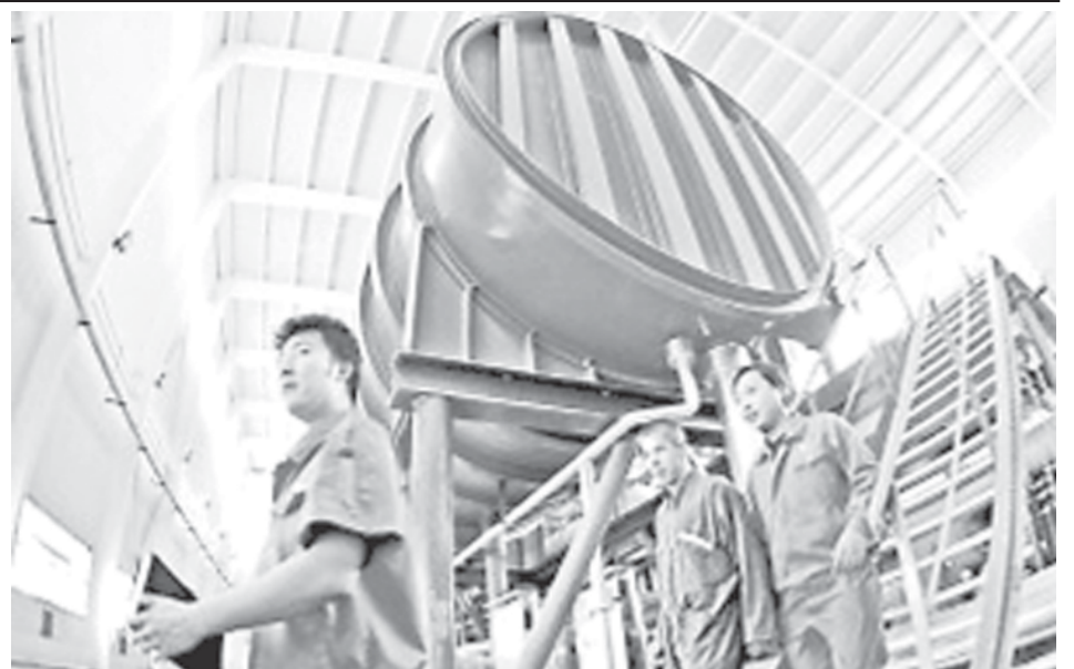
China’s first ten-thousand-ton-class sea water desalting plant has settled in Tianjin Municipality on May 23, 2007. The technology used in the plant is introduced from a French company by Tianjin Baochen Group. The plant will be put into production by the end of this year.—INTERNET
