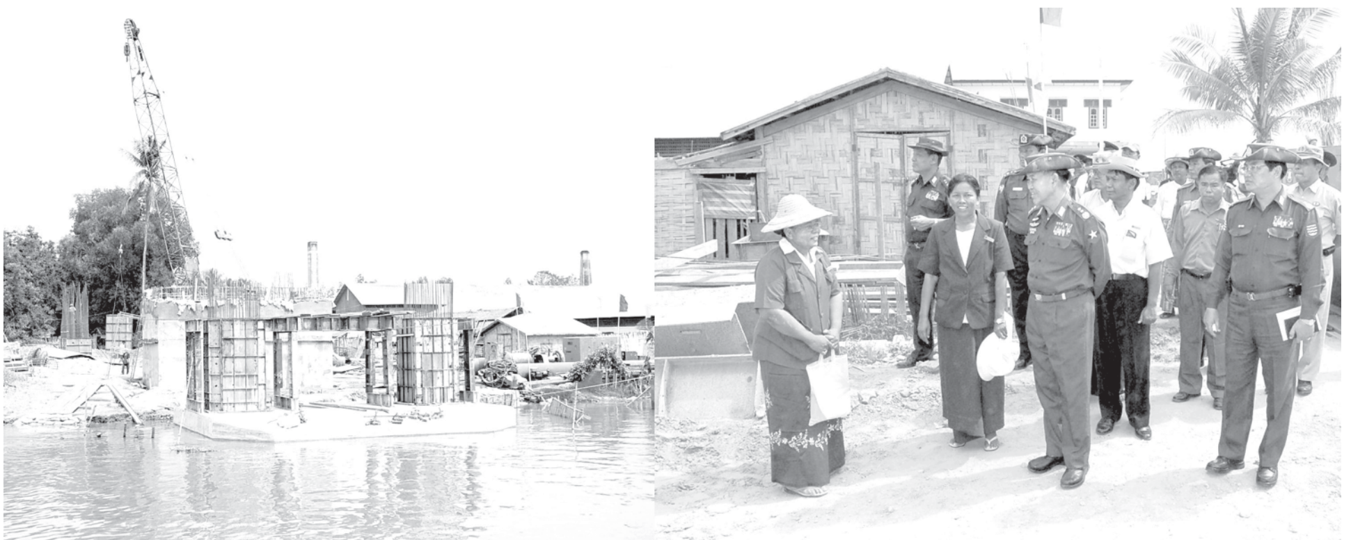
Lt-Gen Khin Maung Than of Ministry of Defence inspects progress of Kyungon Bridge in Wakema. —MNA
