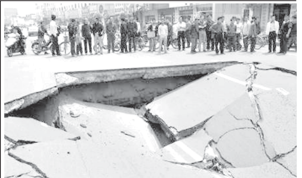
People look at a collapsed section of Shunwai Road in Nanchang, capital of central China's Jiangxi Province on 25 April, 2007. — INTERNET
