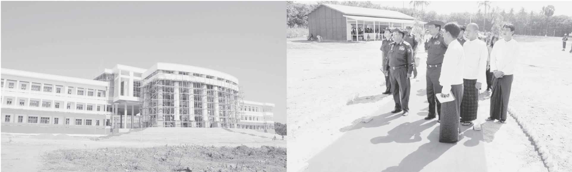
Lt-Gen Maung Bo of Ministry of Defence inspects construction of main building for Technological University in Mawlamyine. — MNA
