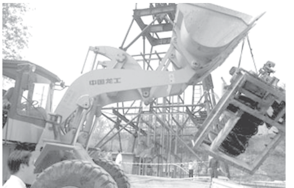
An excavator prepares the rescue work near the pithead in a copper mine pit at Dajipu township of Huangshi city, central China's Hubei Province, on 31 March, 2007. A flooding accident happened in the mine at about 1:00 am Saturday when 21 miners were working underground. Six miners were trapped when the mine was flooded and other 15 miners managed to escape. At present, the rescue work is underway. — XINHUA
