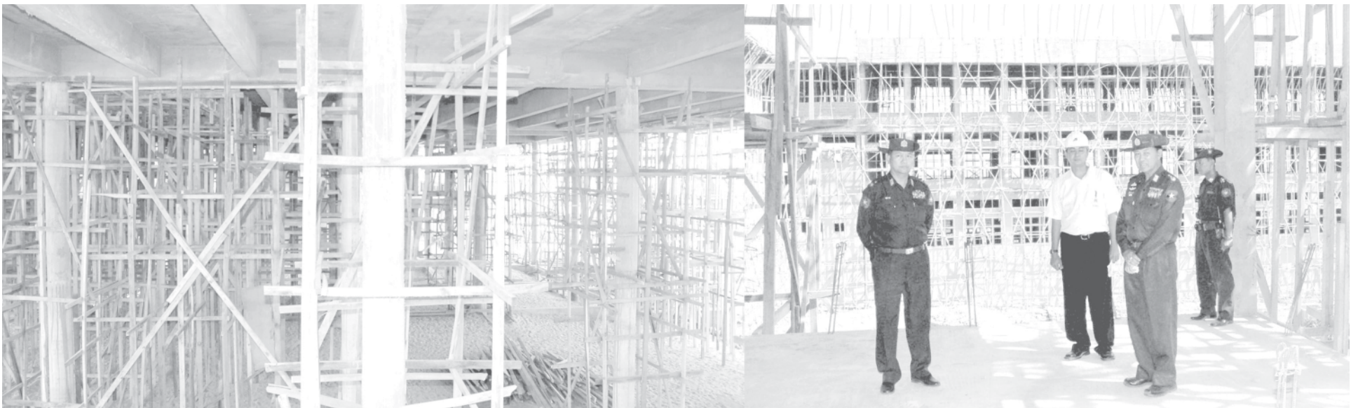
Lt-Gen Khin Maung Than of Ministry of Defence inspects construction of Government Technological College (Toungoo).— MNA
