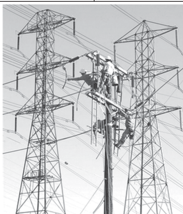
Southern California Edison workers repair power lines in Commerce, Calif, on 28 March, 2007, damaged in Tuesday's wind storm. Workers said it could take up to four days to repair the 12 power poles and four transmission towers effected by the weather. — INTERNET
