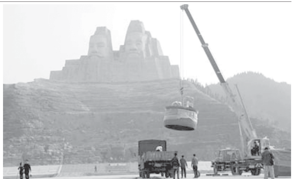
The last tripod is discharged from the truck recently. With the settlement of all nine tripods which symbolize unification of the Chinese, the project of Yan Huang Plaza is to complete. — INTERNET
