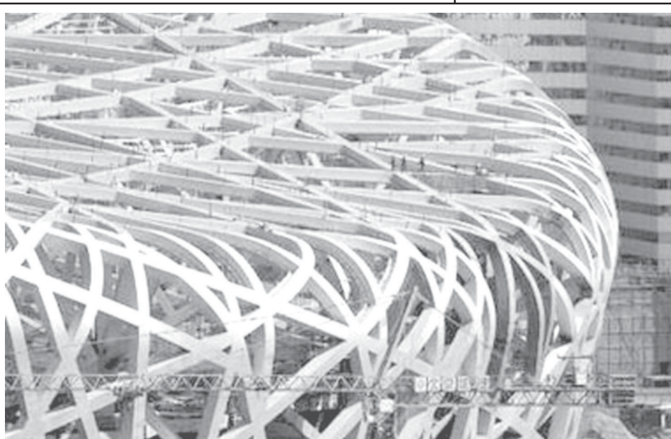
Workers walk at the construction site of the National Olympic Stadium, also known as the 'Bird's Nest', in Beijing, on 27 March, 2007.
