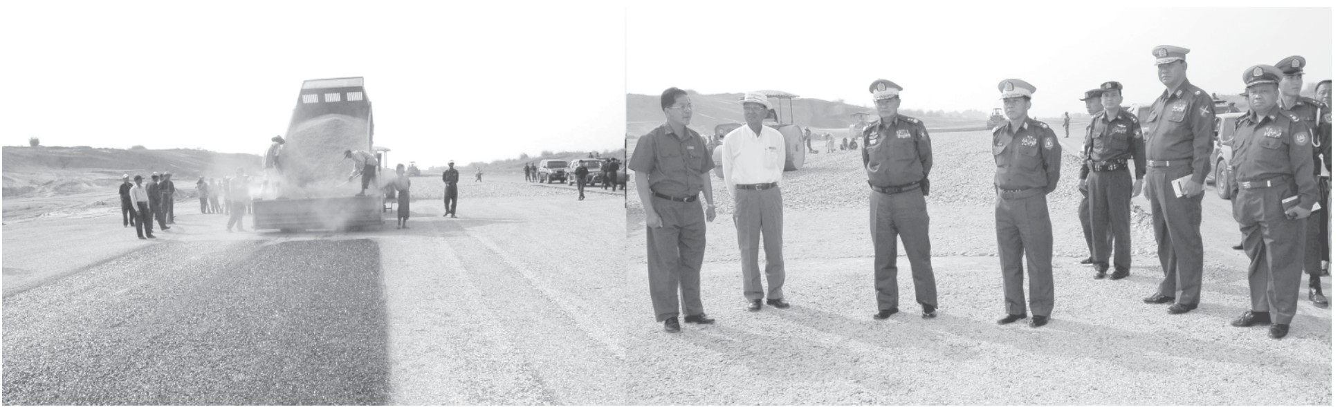
Lt-Gen Kyaw Win inspects extension of runway of Kengtung Airport in Shan State (East). — MNA
