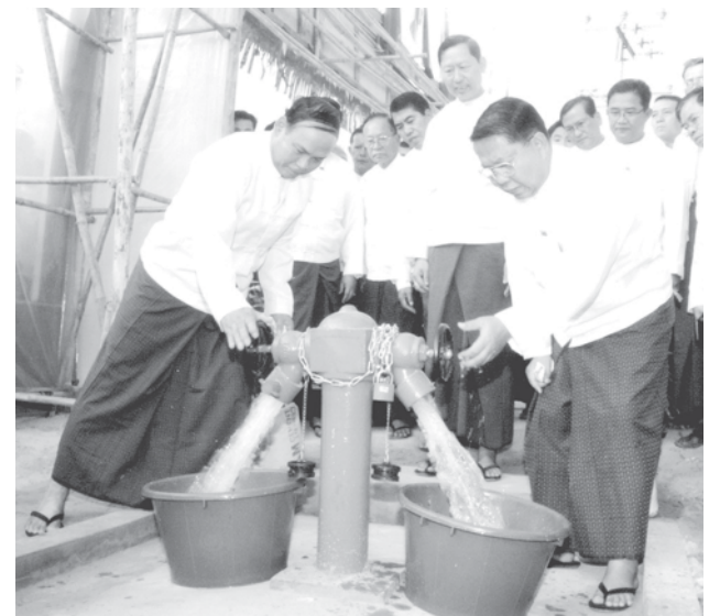
Mayor Brig-Gen Aung Thein Lin and Vice-Mayor Col Maung Pa open the taps of Gyobyu water pipe line in Shwepaukkan. — YCDC
